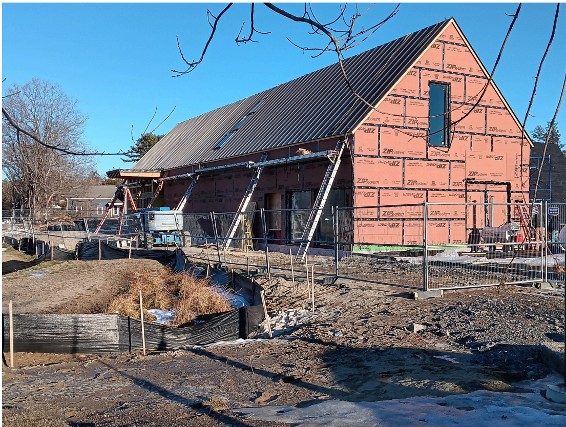
The Ann and Jim Hancock Education Center is one of two buildings under construction at Maine Audubon's Gilsland Farm in Falmouth. PHOTO / TINA FISCHER
